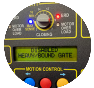
Heavy gate or binding gate detected
